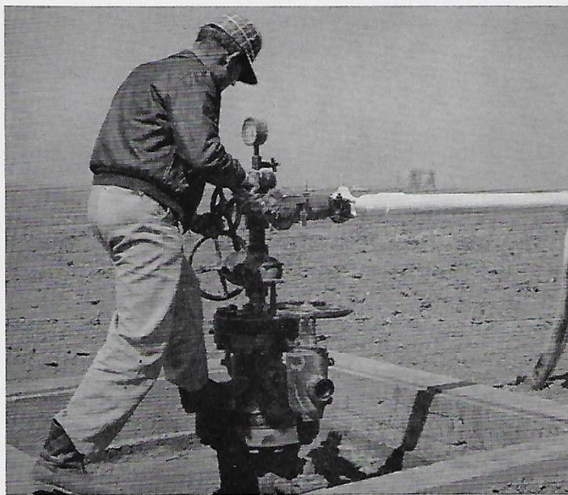
Union No. 1 Luthi in the Texas Panhandle was brought in during February, 1956. It has tested 884 barrels of oil daily on a half-inch choke. Engineer Don Holland is holding it back to the Texas allowable of 101 barrels daily, 16 days per month. Frost on the pipe is evidence of the reduced well-head pressure.
